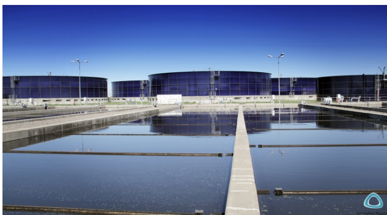
Picture 16 Adlia wastewater treatment plant
