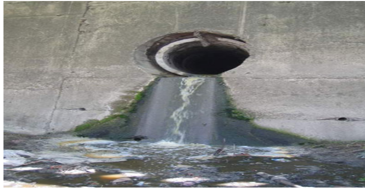
Picture 4 The waste water of treatment plant
