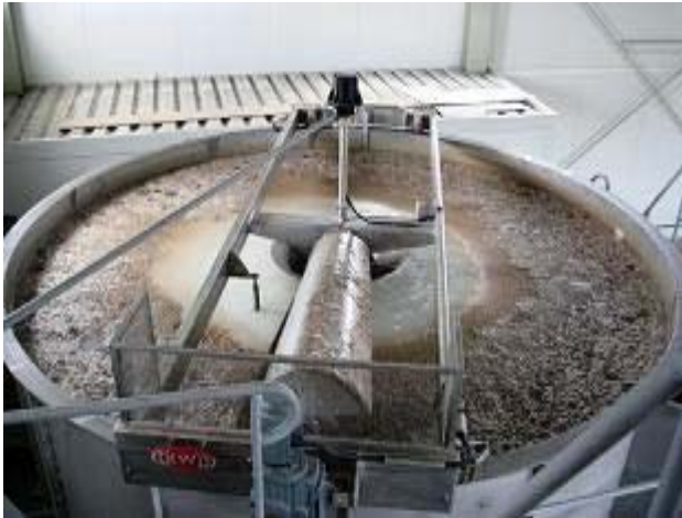
Picture 8 Picture 9 Flotation device
